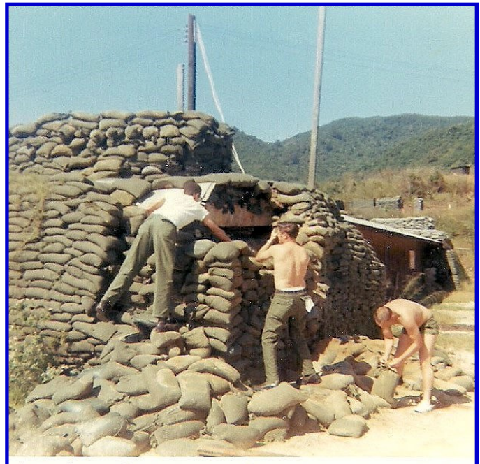
ELD4 crew of (L-R) BM1 Holman, GM1 Padgett, and BM1 Hicks conducting “home improvement” on defensive bunker at ELD4 compound.
